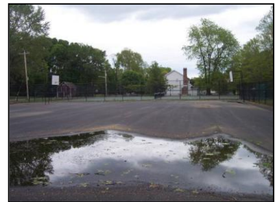
Drainage issue at Locust Lane Park
