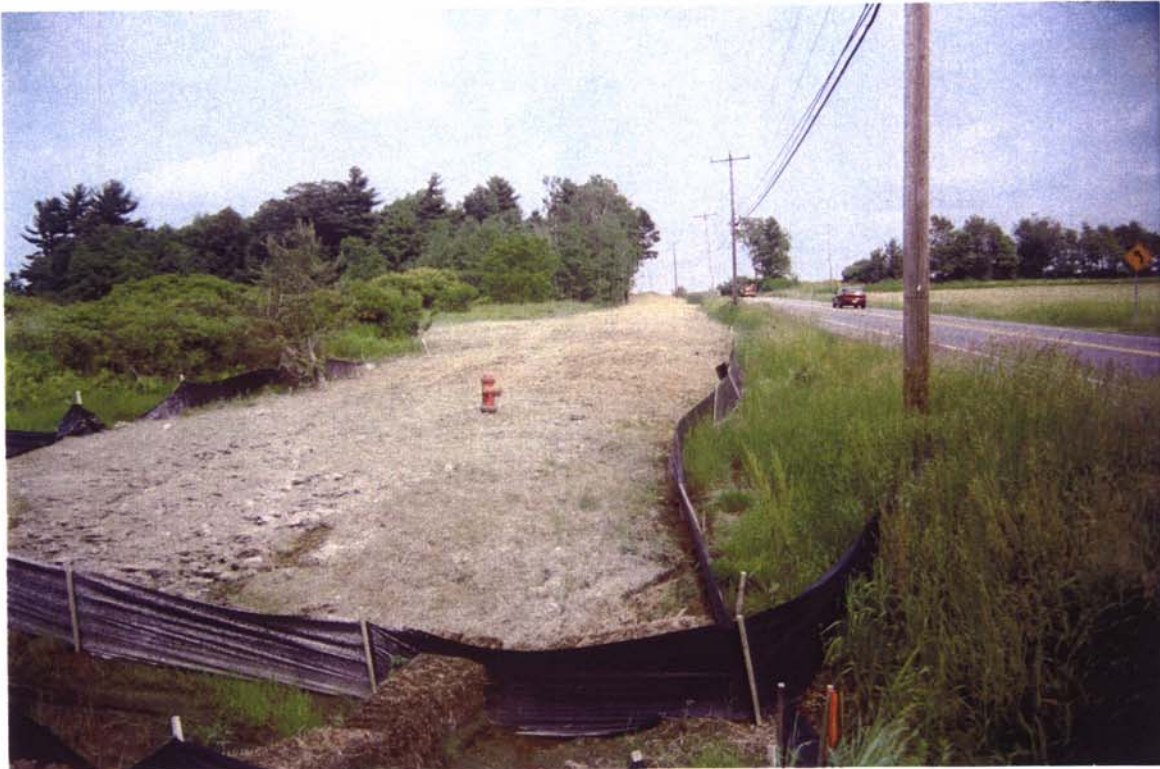
14. East view of recent disturbance from the placement of a water line on the north side of NY Route 146.
