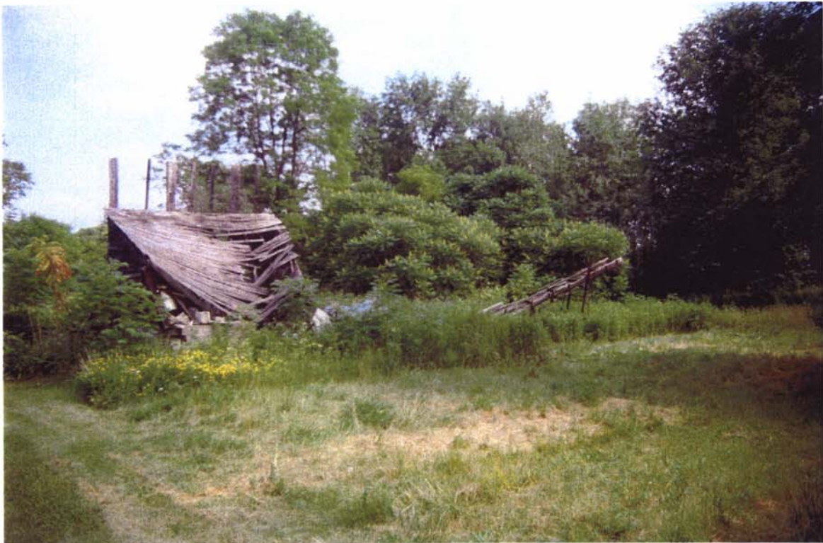
12. Southeast view of collapsed outbuildings on the south side of NY Route 146A.
