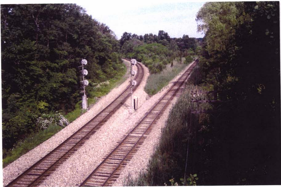
16. Northwest view of two branches of the Delaware and Hudson railroad along Ashdown Road.
